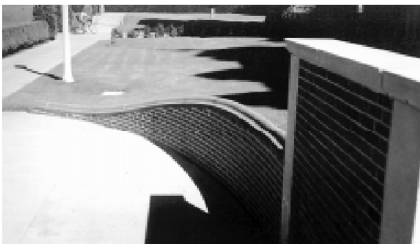
Wall Photograph B, Student Union.
