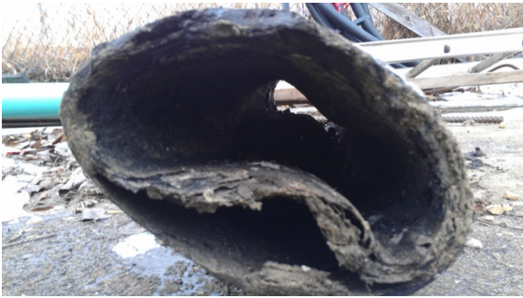
Figure 37, Failed Orangeburg Electrical Conduit
