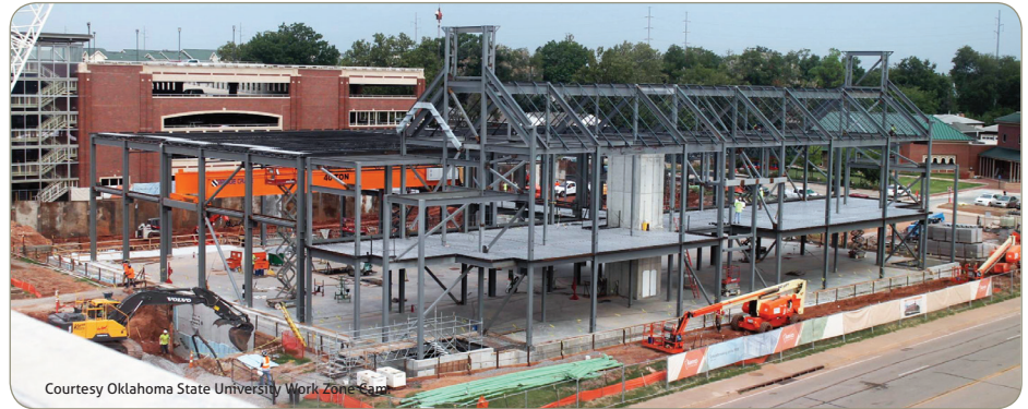
Courtesy Oklahoma State University Work Zone Team Construction of OSU's new Central Plant, for which ground was broken in fall 2015, is under way with service to campus expected to begin in December 2017.
