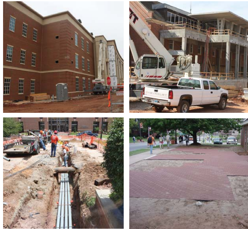
Construction is an important part of the process to transform planning concepts into completed projects that can be enjoyed.
