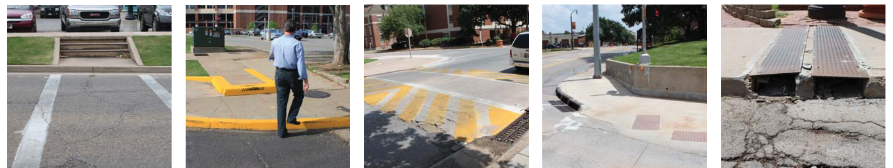
Improvements are needed in many areas to address accessibility and general maintenance issues.
